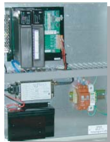
View into an upgraded waste water pump station RTU cabinet
